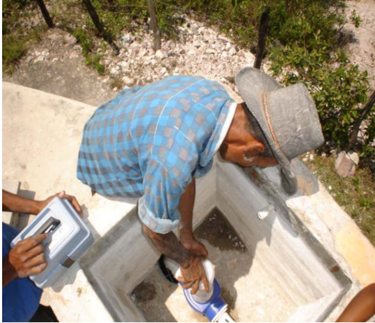
Community plumber, Cristiano, checks the chlorine level in the community water system.
